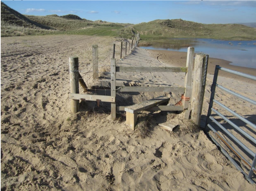
Photograph 17. Sand accumulation on the eastern side of the haul road, northern end of the Phase II area
